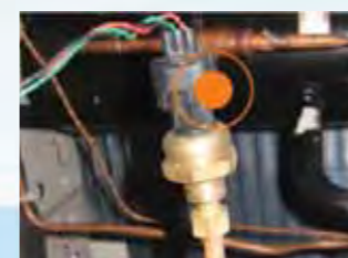
Always test the system pressure
