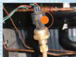
Always test the system pressure
